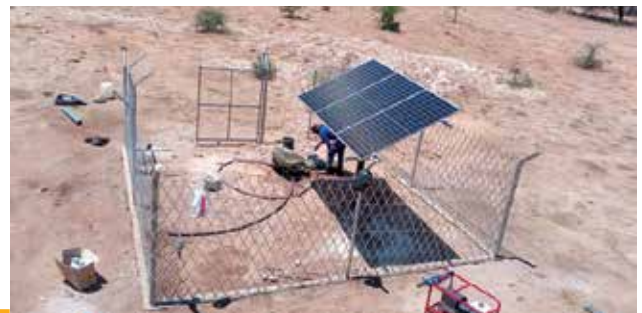
Enclosed solar system and borehole with fence.
